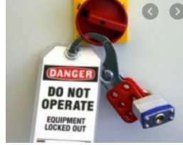
Fig. Error! No text of specified style in document..3 Electrical Lock-out system
