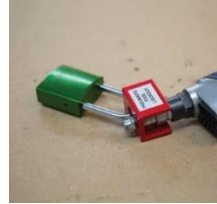
Fig. Error! No text of specified style in document..4 Pneumatical Lock-out system
