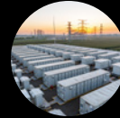
Power & Data Infrastructure
