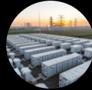
Power & Data Infrastructure
